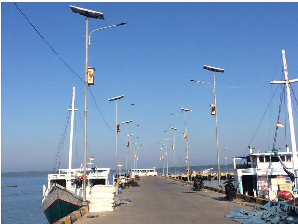
Figure 4. Solar powered streetlight at Benteng port
