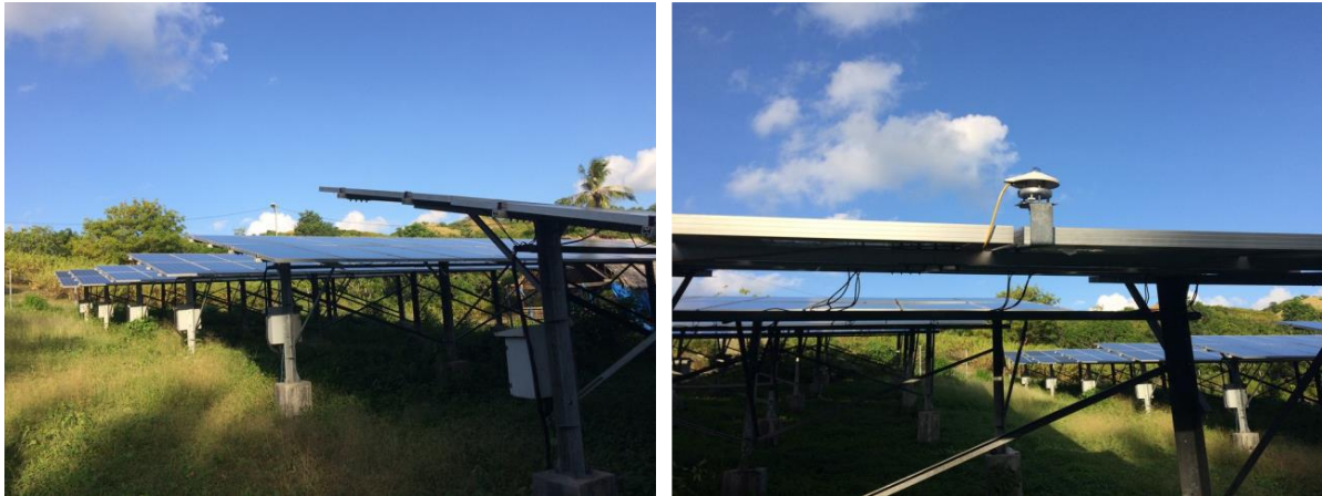
Figure 3. Existing solar farm on Tambolongan Island
