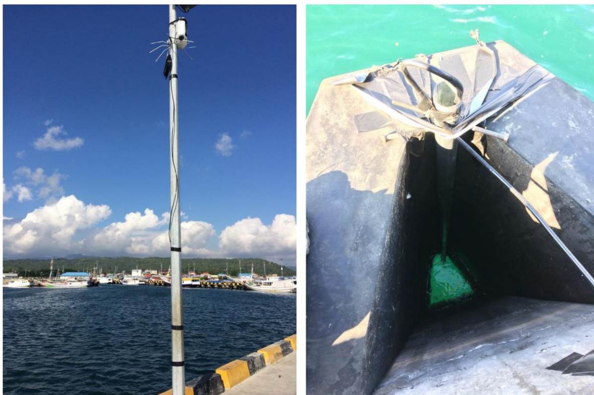
Figure 1. Tide gauge installation at Benteng port
